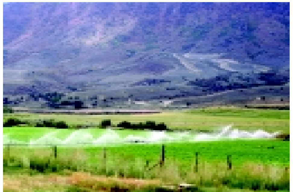
Sideroll sprinkler, one of many conservation measures, installed on West Elk Ranch.
